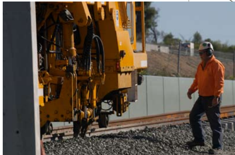
Track-laying along the 72km route of the Southern Suburbs Railway progressed rapidly.
