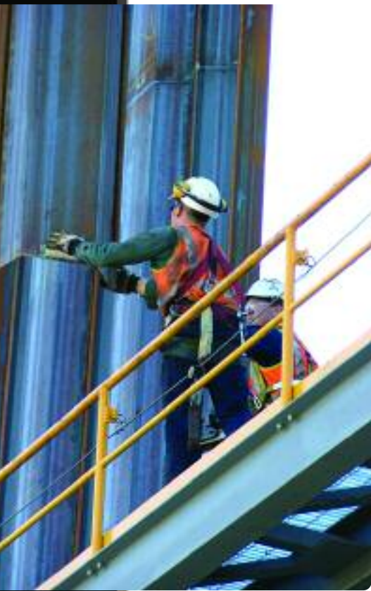
Work under way on the city component of the New MetroRail project.
